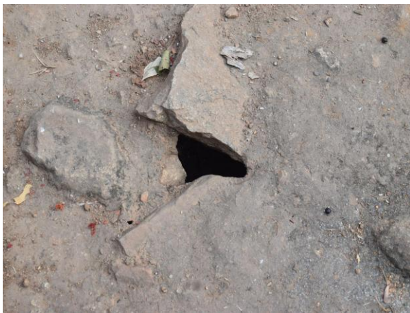
Underground holes and gaps
