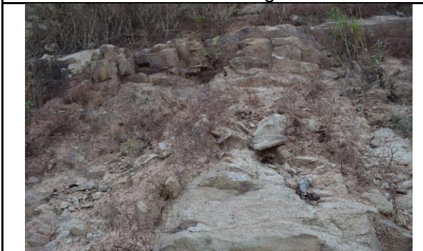
Loose rocks and soil-filled areas on the vertical
